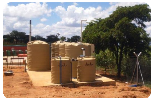
Water treatment station
